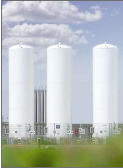
AC SCS.1 Line Vertical Bulk Tanks
