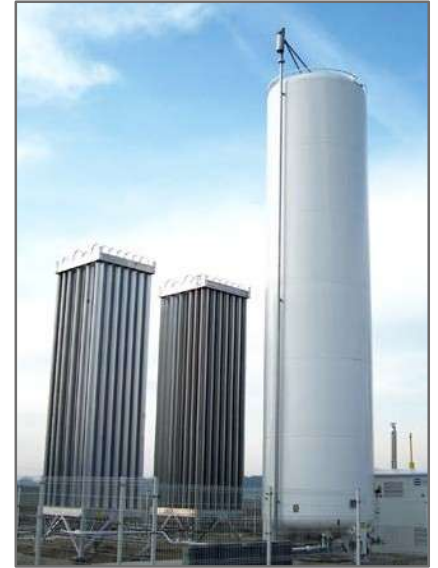
AC SCS-LNG Line Bulk Tanks
