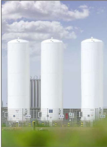
AC SCS.1 Line Vertical Bulk Tanks
