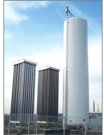
AC SCS-LNG Line Bulk Tanks
